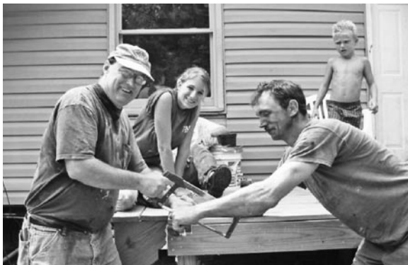
Volunteers and clients work together on construction. Image courtesy of the Author.
